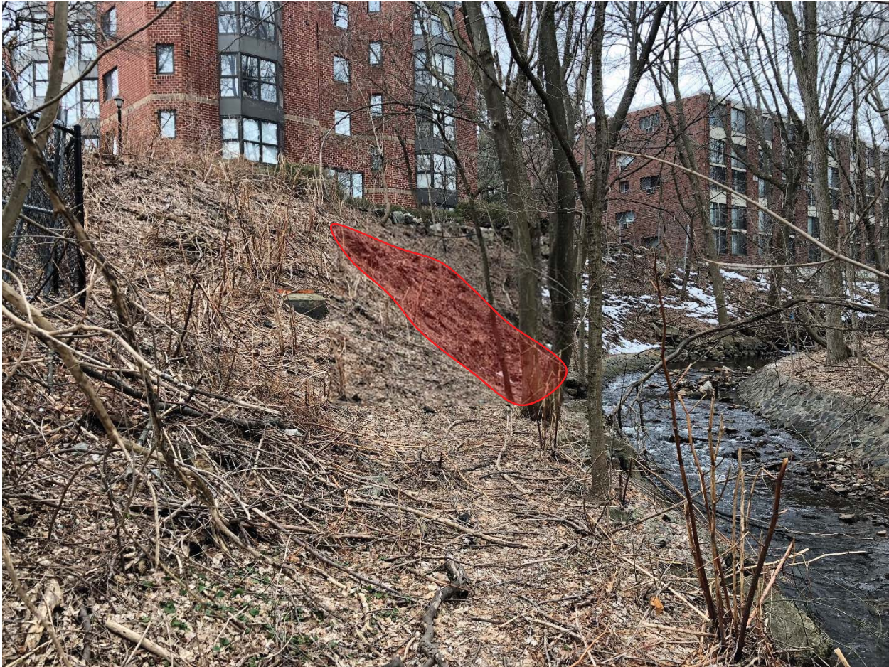
Photo 5: Looking west toward "Erosion-1A". (Private property)
