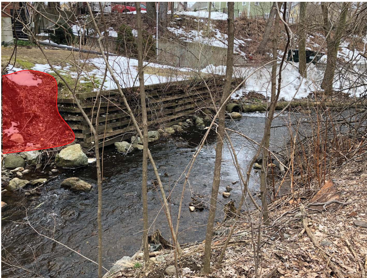
Photo 8: Looking south-west; “Erosion-2B” adjacent to “living wall”. (Private property)
