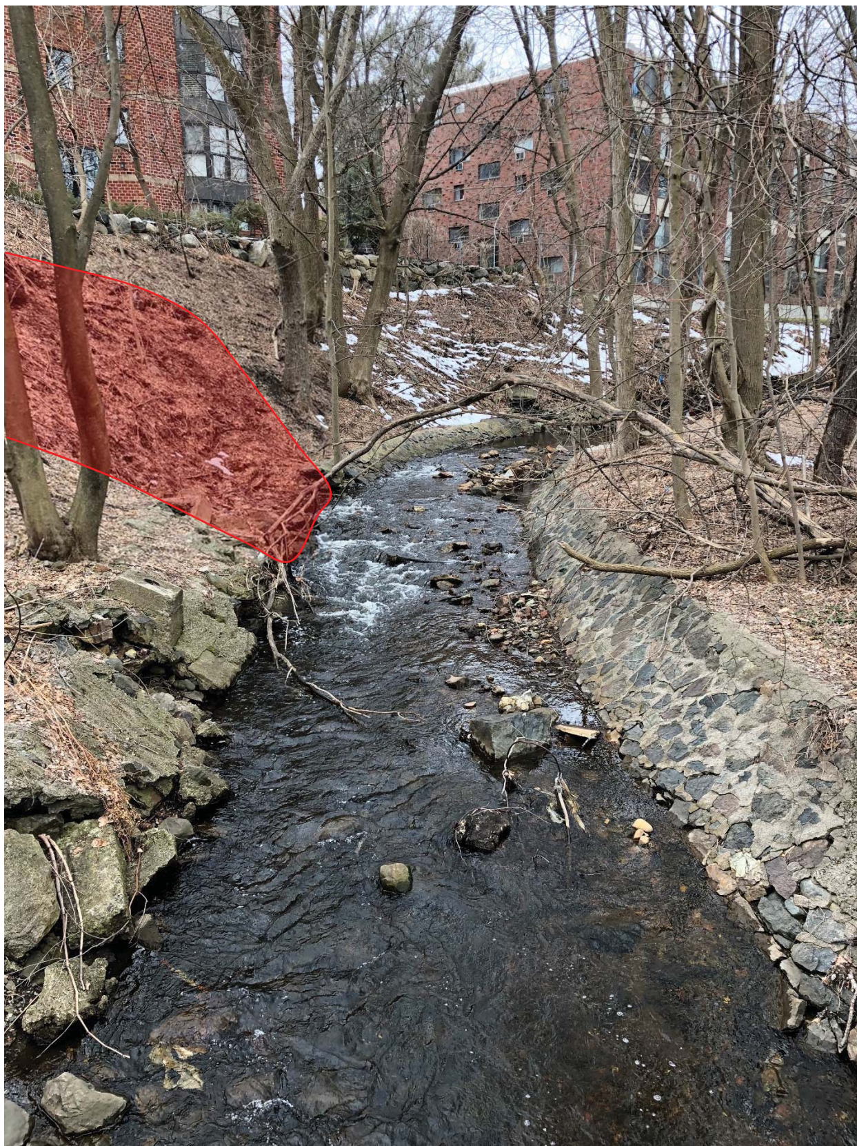
Photo 6: Looking west toward south bank and “Erosion-1B”. (Private property)
