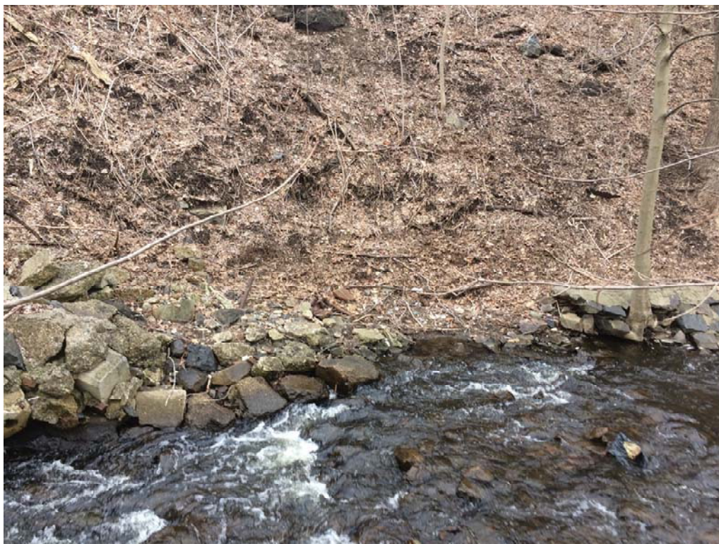
Photo 3. Erosion area west of bridge, southern bank. (Private property)
