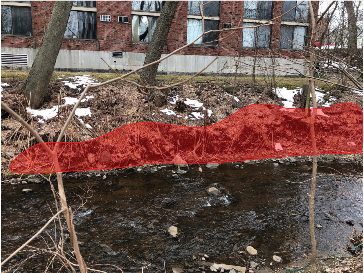
Photo 7: Looking south toward south bank and “Erosion-2A”. (Private property)
