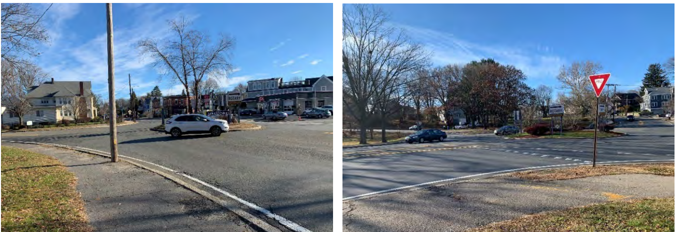
Figure 17 (Left) Excess pavement and lack of horizontal deflection at the High Street rotary; (right) no crossing on the path side of the Medford Street rotary
